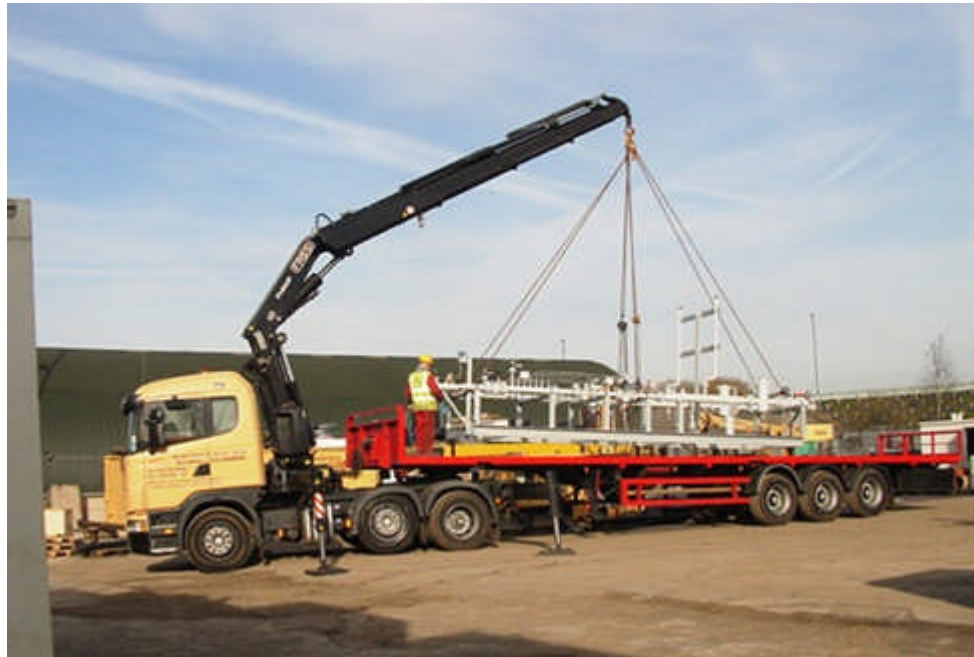
Pictured above: Rayden Transport loading gas pressure reduction unit manufactured at Ilkeston depot 2009
